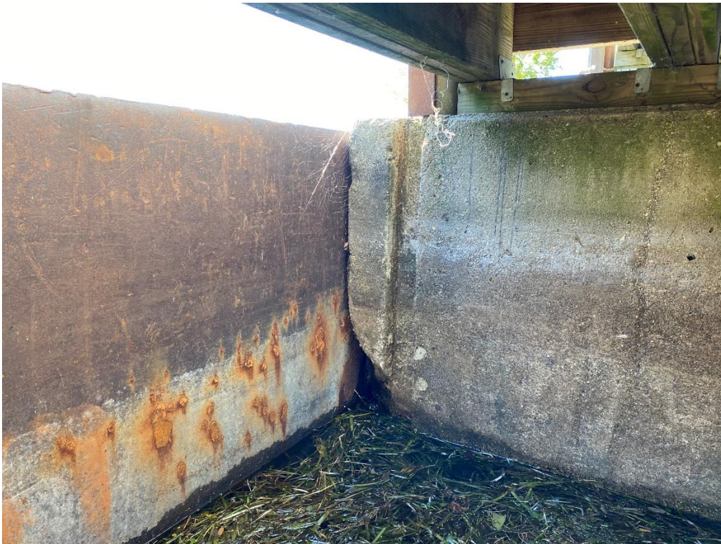
Spillway Bay, 4 th From Left. Note Damaged Concrete, Left Side of Bay
