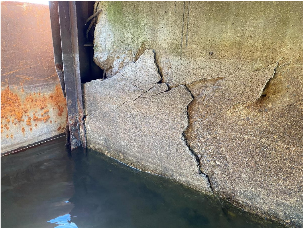
Other Side of Bad Pier
