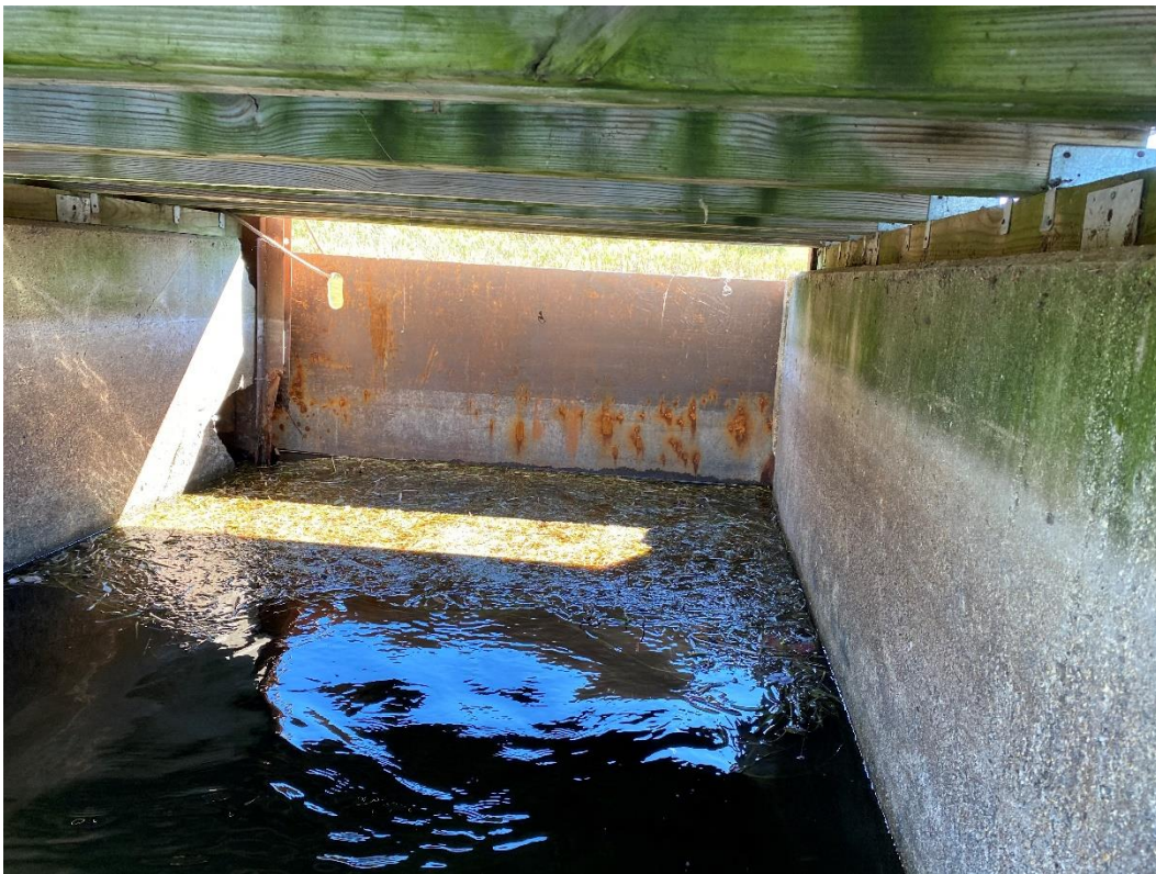
Spillway Bay, 4 th From Left. Note Steel Plate for Lake Control & Bad Pier
