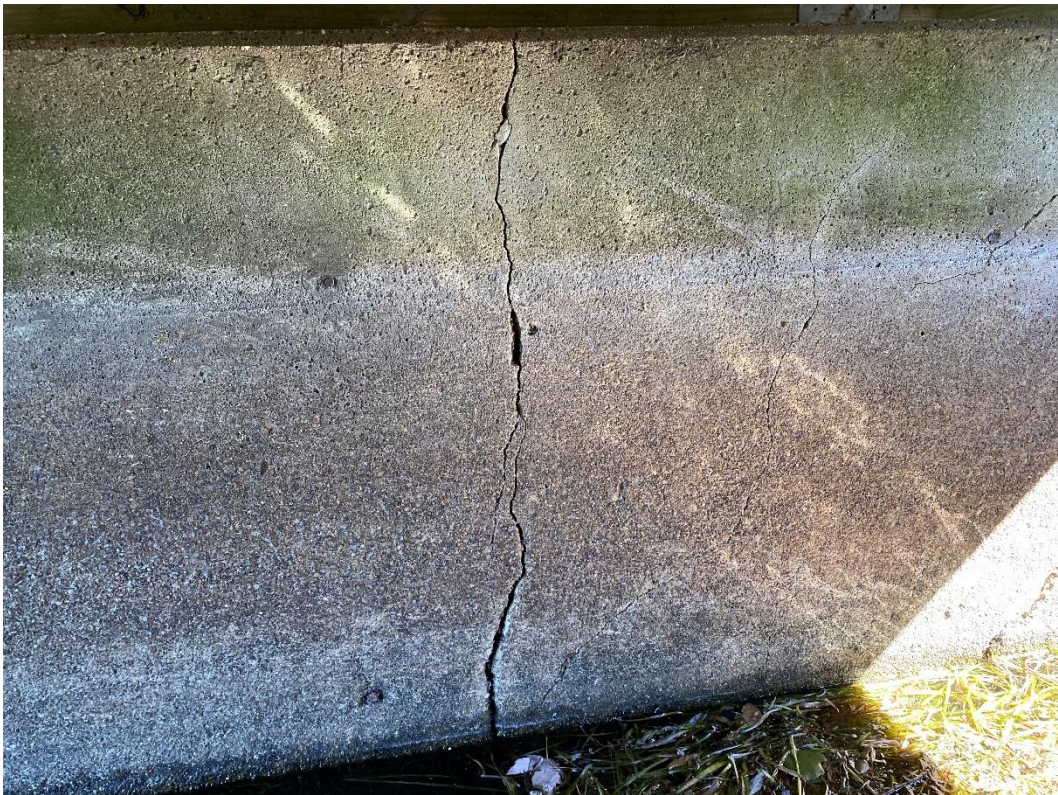
Crack in Same Pier
