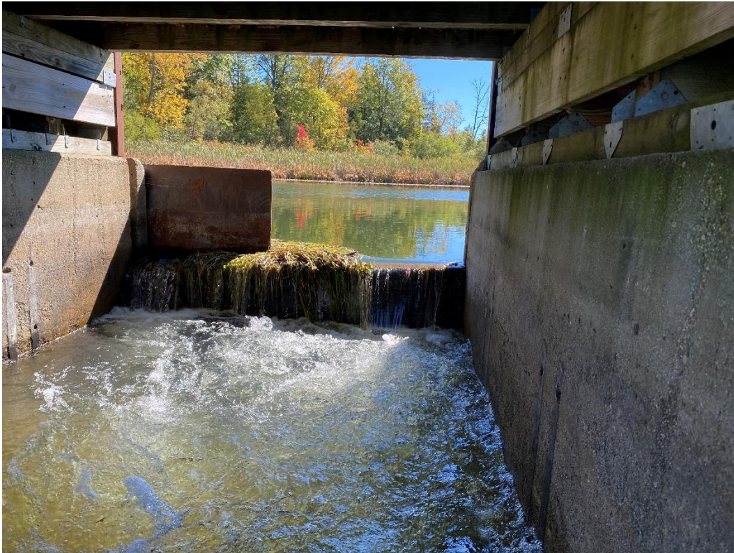
Spillway Bay, 3 rd From Left. Note Steel Plate Used for Adjacent Bays
