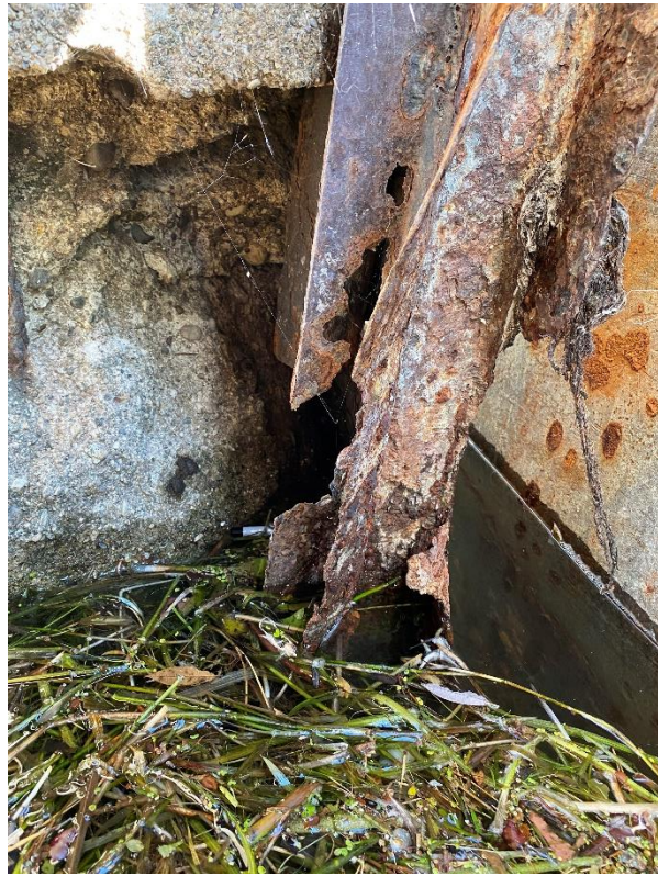
Badly Corroded Gate Channel
