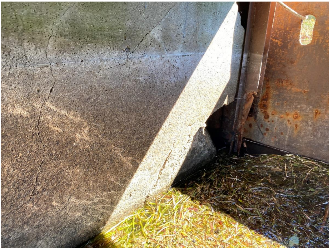
Close Up of Bad Pier, Right Side of Bay
